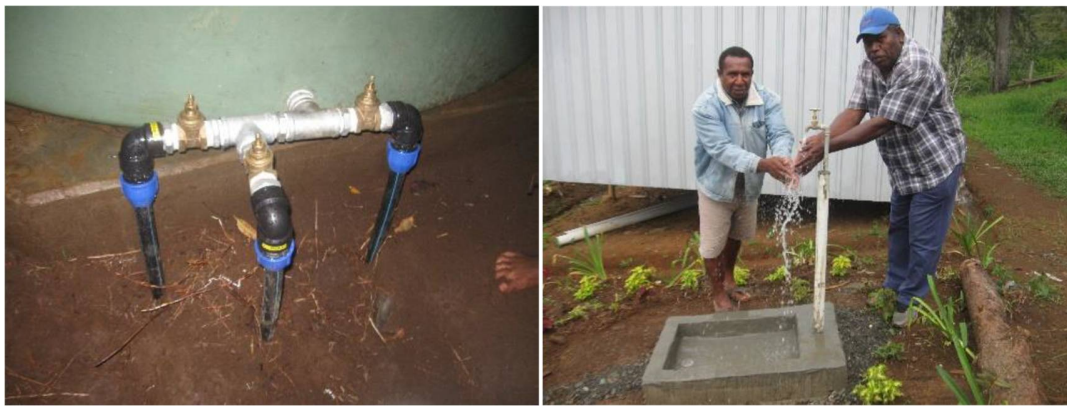
Photo on right: 9000L tank with three parallel lines hooked up. The first service line supplies the community. The second line supplies the health centre and health staff residence. The final line supplies the elementary school including the hamlets along the way.
