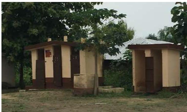
Missing and Broken Doors on Structures
