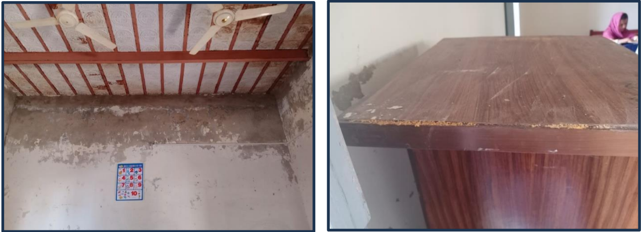
Picture 5: School condition after recent monsoon rain
