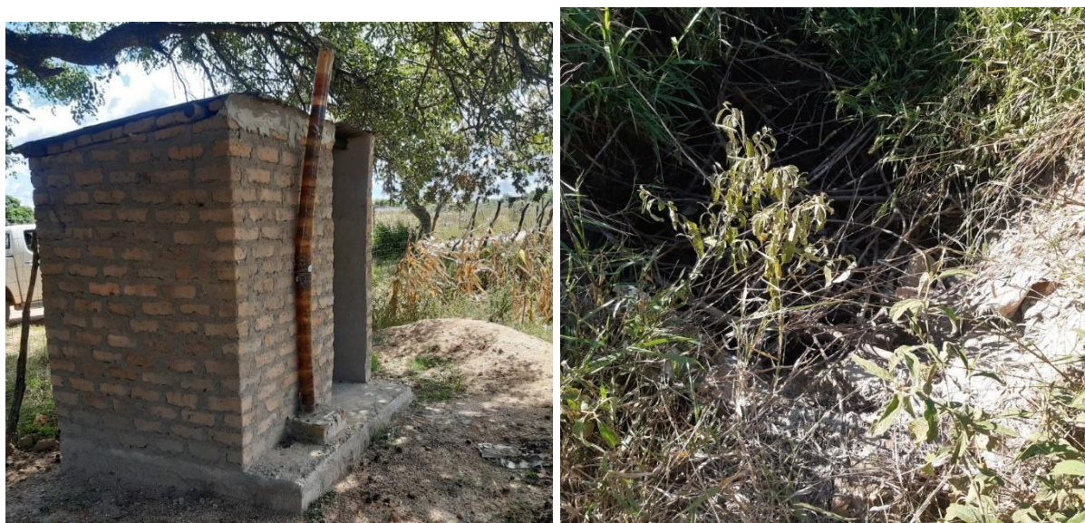
Plate 3: a) An improvised vent pipe from locally available materials b) Latrine constructed from local material destroyed by extreme weather event
